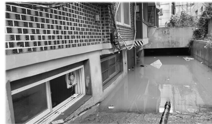
A semi-basement house in Sillim-dong was flooded by record-breaking heavy rain in August 8, 2022.
